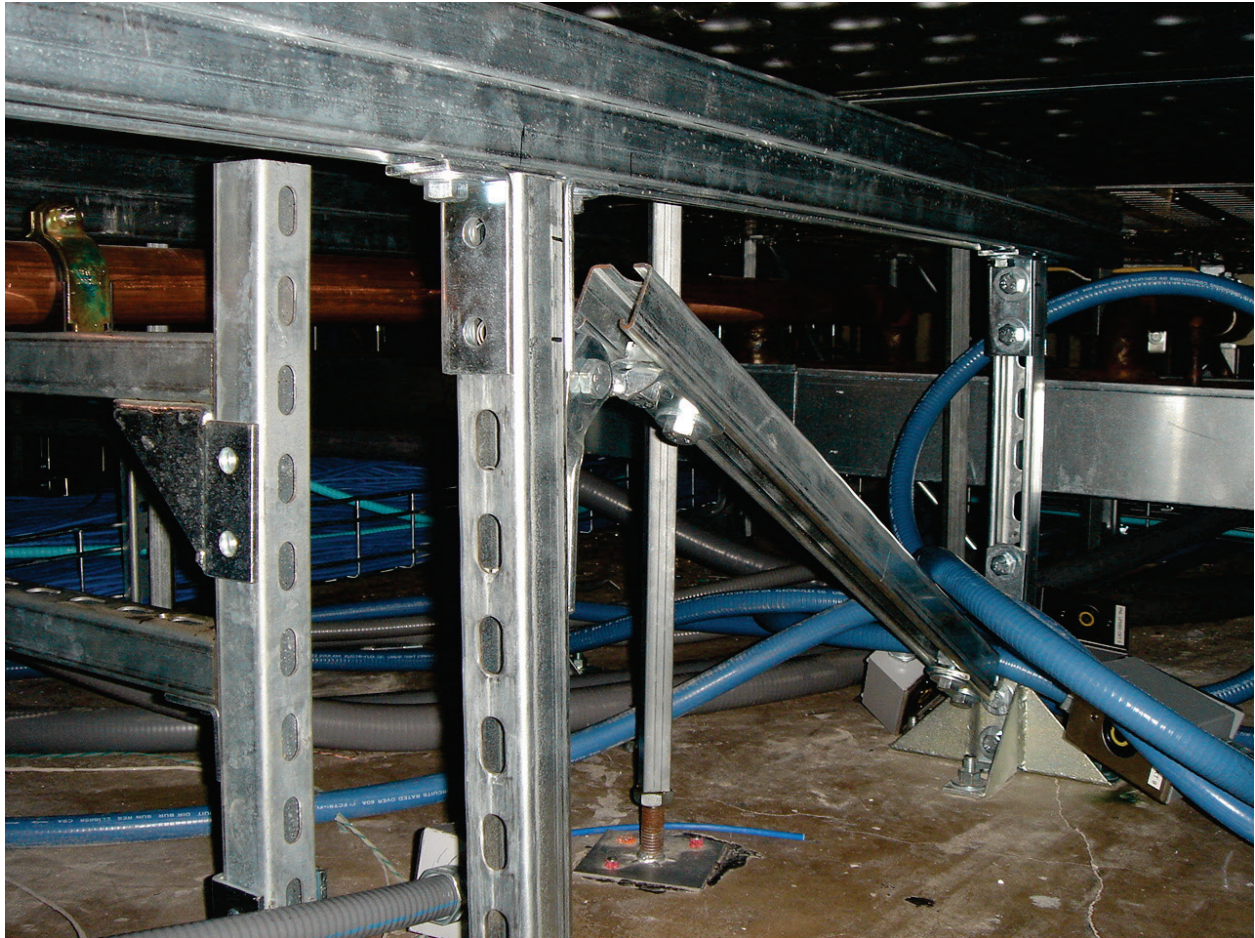
Figure 6.5.3.1-8 Strut framing added to brace data cabinet located on access floor. Bolts from angles above are connected to strut framing below (Photo courtesy of Maryann Phipps, Estructure).
