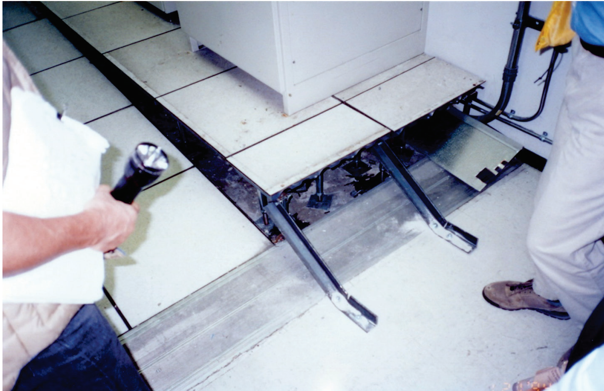
Figure 6.5.3.1-1 Temporary bracing for access floor collapsed in the 1994 magnitude-6.7 Northridge Earthquake (Photo courtesy of Wiss, Janney, Elstner Associates).
