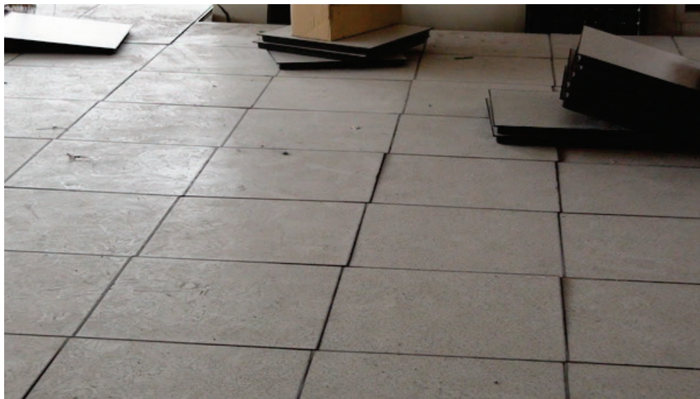
Figure 6.5.3.1-2 Damage to access floor with short anchored pedestals in the 2010 magnitude-6.7 Chile Earthquake; floor did not have lateral bracing. Note many tiles misaligned (Photos courtesy of Antonio Iruretagoyena, Rubén Boroschek & Associates).
