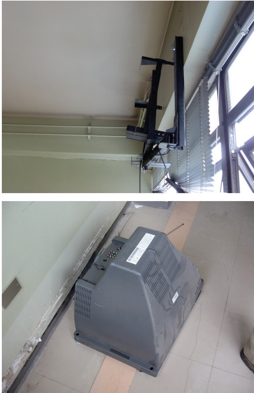
Figure 6.5.3.4-1 Wall-mounted monitor fell from the bracket in a hospital in the 2010 magnitude-8.8 Chile Earthquake; bracket still anchored to the wall (Photos courtesy of Rodrigo Retamales, Rubén Borosc hek & Associates)
