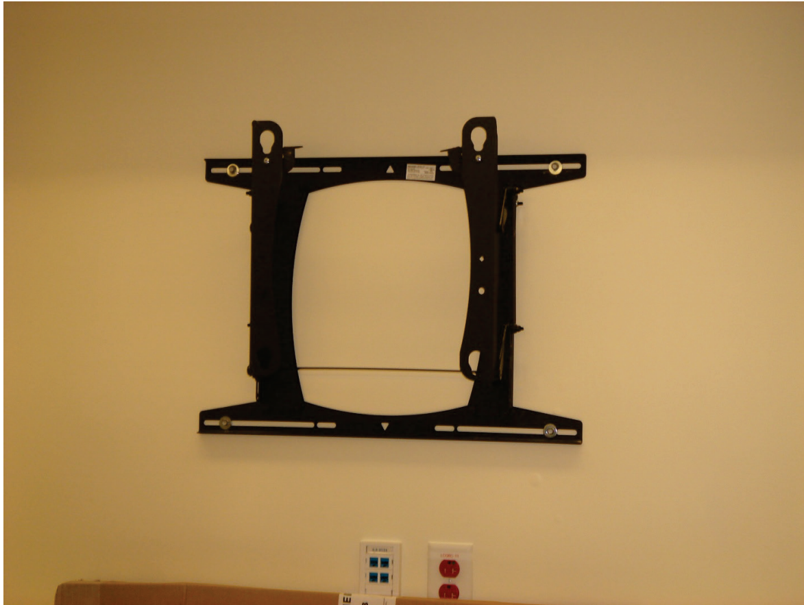
Figure 6.5.3.4-2 Wall-mounted television bracket anchored with sheet metal screws to wall studs at four locations. Bracket must be rated for the weight of television or monitor and that the unit must be securely attached to the bracket (Photo courtesy of Maryann Phipps, Estructure).
