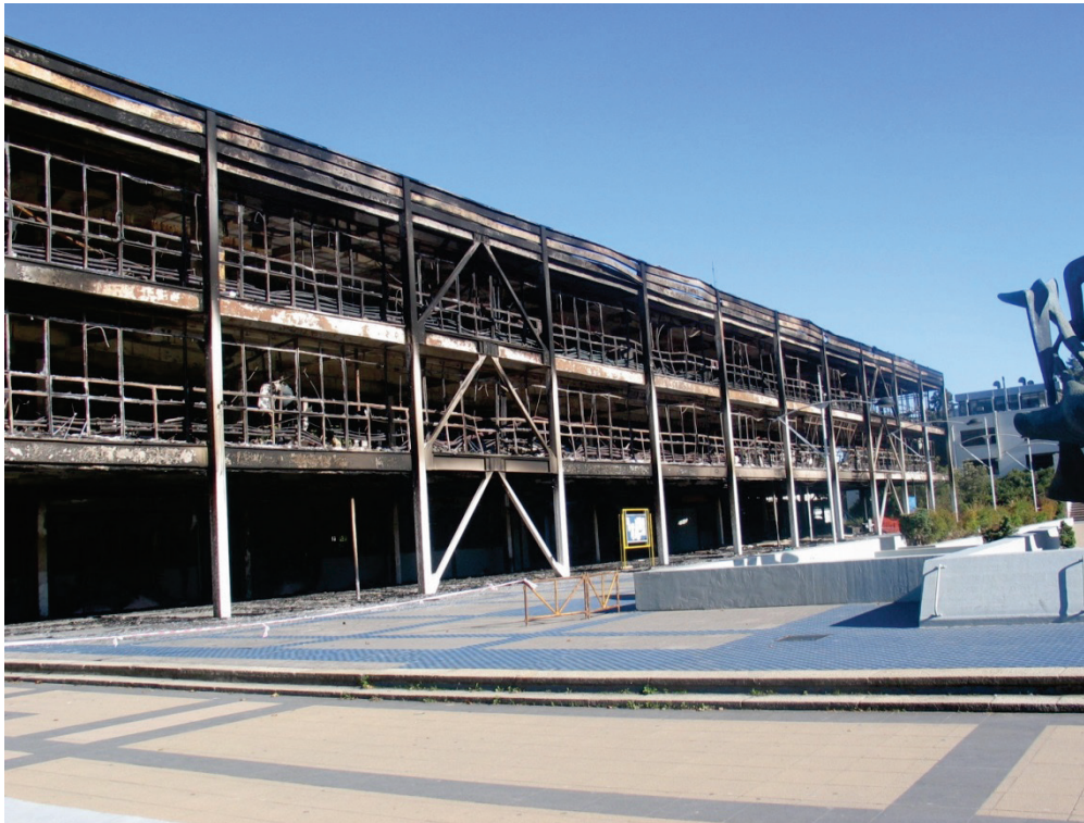
Figure 6.5.4.1-4 Fire destroyed the chemistry building containing the entire chemistry department at the University of Concepción in the 2010 magnitude-8.8 Chile Earthquake; fire exacerbated by the presence of hazardous chemicals (Photo courtesy of Bill Holmes, Rutherford & Chekene).
