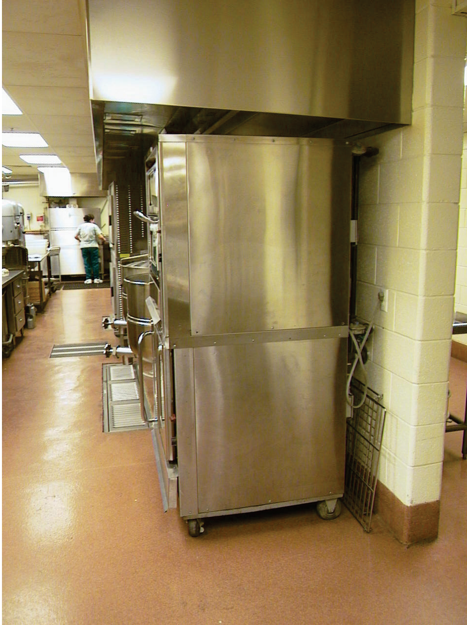
Figure 6.5.5.3-2 Existing condition: Unrestrained kitchen equipment (Photo courtesy of EQE for the Salt Lake City School District).
