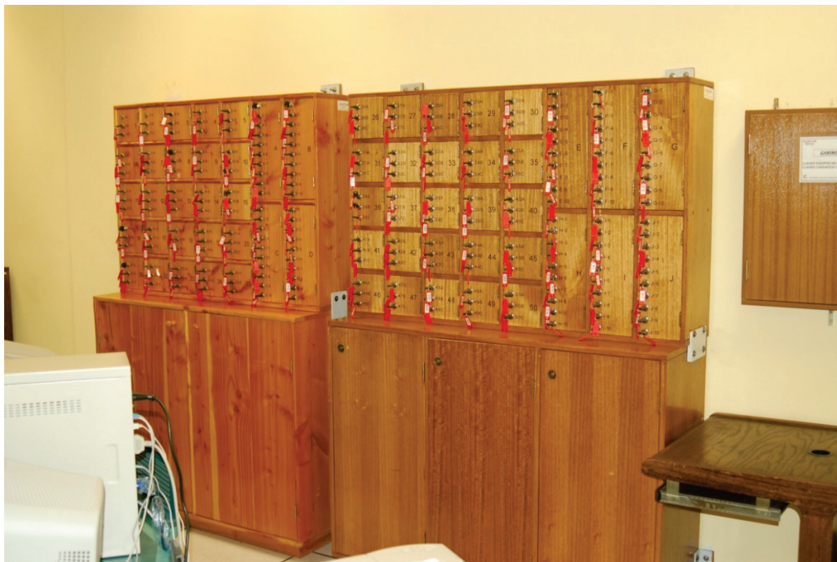
Figure 6.5.5.3-4 Anchored wood key cabinets in industrial plant control room; note top and bottom units anchored together and both anchored to wall (Photo courtesy of Eduardo Fierro, BFP Engineers).
