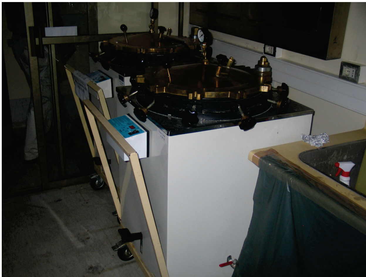
Figure 6.5.5.3-3 Equipment on wheels did well during the 2010 magnitude-8.8 Chile Earthquake; there were no reported injuries or examples of overturning related to equipment mounted on wheels. Centrifuges on wheels shown in photo (Photo and information courtesy of Bill Holmes, Rutherford & Chekene).
