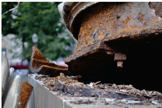
Figure 6.5.6.3-2 Leaning fountain after the 2010 Chile Earthquake; corrosion was a factor (Photos courtesy of Eduardo Fierro, BFP Engineers).
