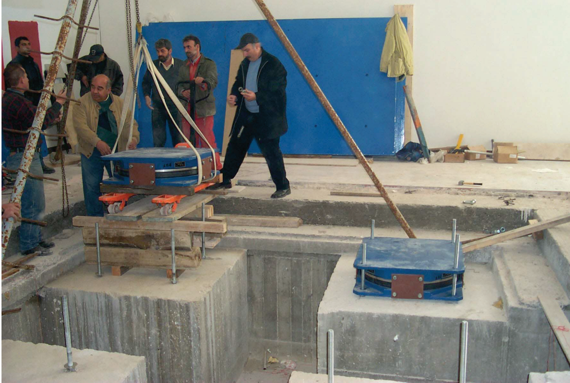
Figure 6.5.6.3-3b Installation of base isolation devices to support reinforced concrete slab for statue (Photo courtesy of University at Buffalo).
