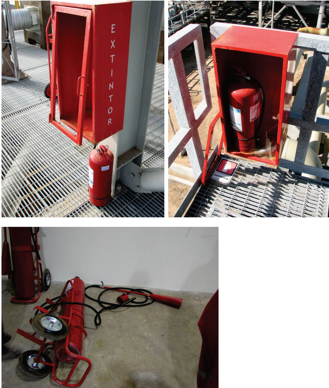
Figure 6.5.6.4-1 Fire extinguishers damaged during the 2010 magnitude-8.8 Chile Earthquake at an industrial facility (Photos courtesy of Antonio Iruretagoyena, Rubén Boroschek & Associates).
